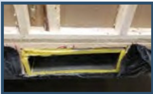
Fiberglass Heat Ducts w/in Floor Cross Over Heat— Standard
